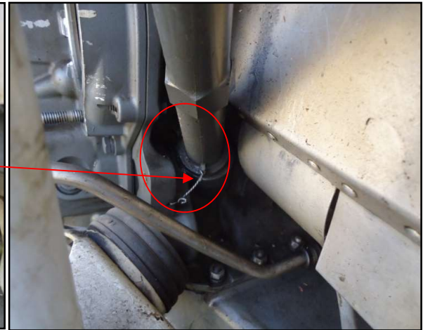
Fig 23: Shift in Oil Filler tube wire lock position
