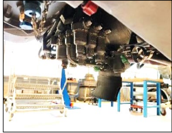
Figure 94 – Drain Collector Assembly Forward View (Undamaged)
